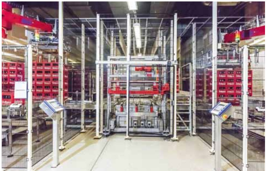
Problem solved: Machinery guidelines with regard to safety are a real challenge for the planning, especially in the case of existing plants with a defined footprint and specified interfaces
